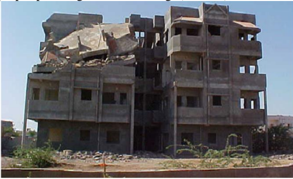
Fig. 1.2: Ground storey collapse of a 4-storey building with plan irregularity at Bhuj. [14]
