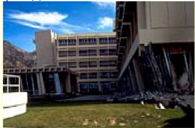
Fig. 1.1: Ground storey collapse of a 4-storey building with open ground storey at 240 Park Avenue South in New York, US. [12]
