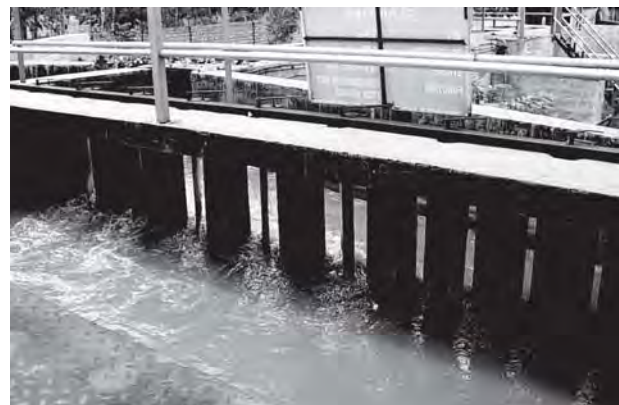
Fig. 18.4 Grit and sand removal tank
