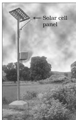
Figure 14.7 A solar cell panel
