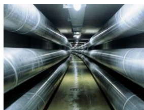
System Length 1 km - Palexpo, Switzerland Underground Part of a GIL/Overhead Line
