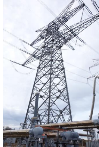
Transition section GIL to overhead line.
