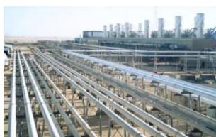
Length 17 km – PP9 Saudia Arabia Longest 420 kV GIL installed in the world
